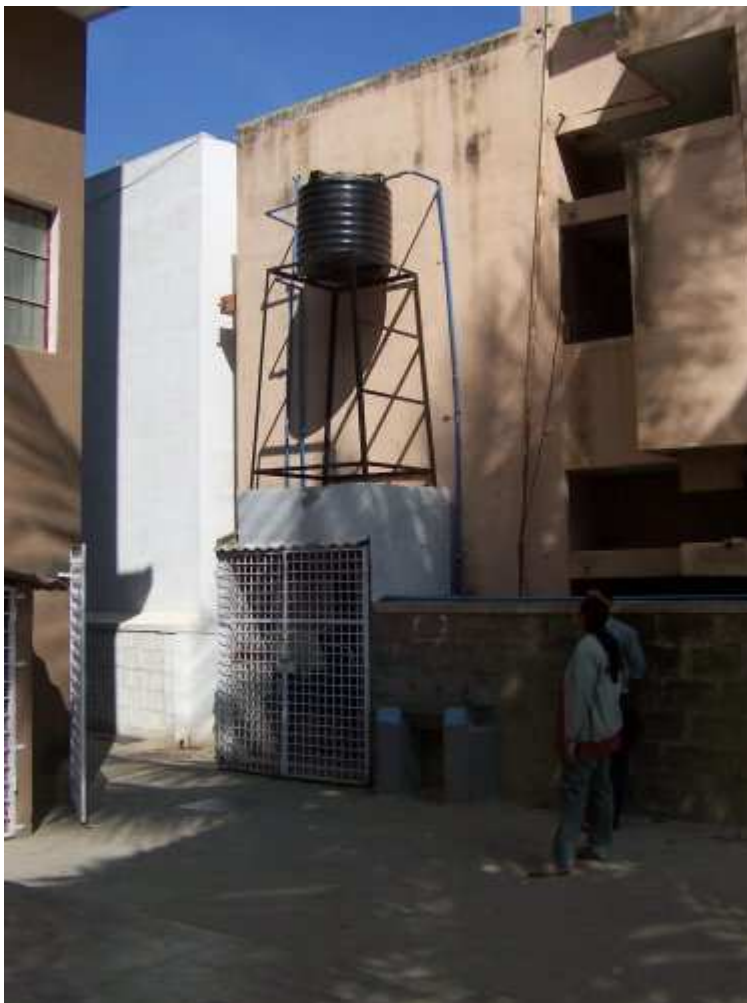
Independent drinking water system
